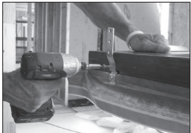
Figure 12. Z bracket installation on a Zola Thermo Wood window. Image courtesy Zola Windows.
