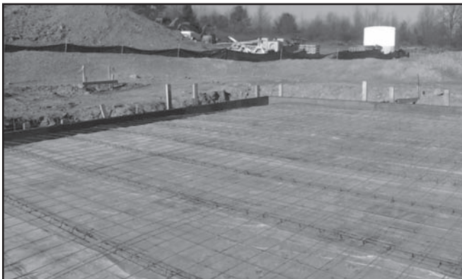
Figure 9. First slab poured 11/2012. There is 5 1/2" of polyisocyanurate insulation under the plastic. Image courtesy Lois Arena. Figure courtesy Kendall Carpenter.
